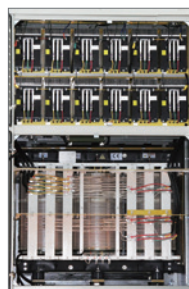
Power cell cabinet (Top) Transformer cabinet (bottom)
